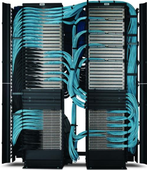
Figure 1. Proper Cable Management
